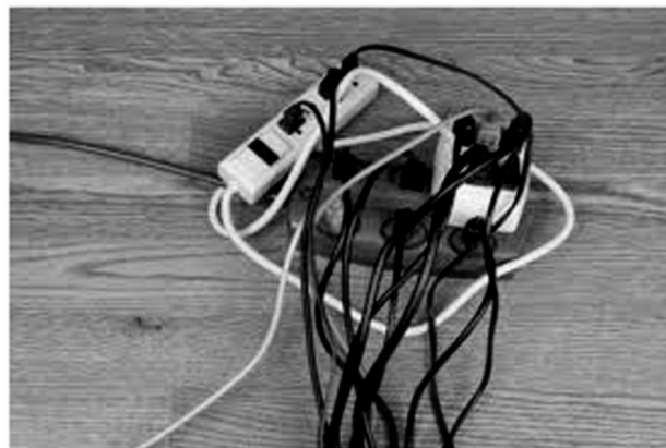
Fig. 11.2: Overloaded power strip.
