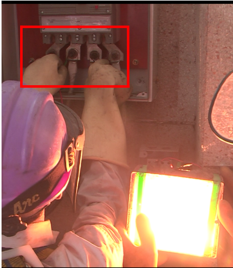
Phase-to-phase checking of sequence 2
