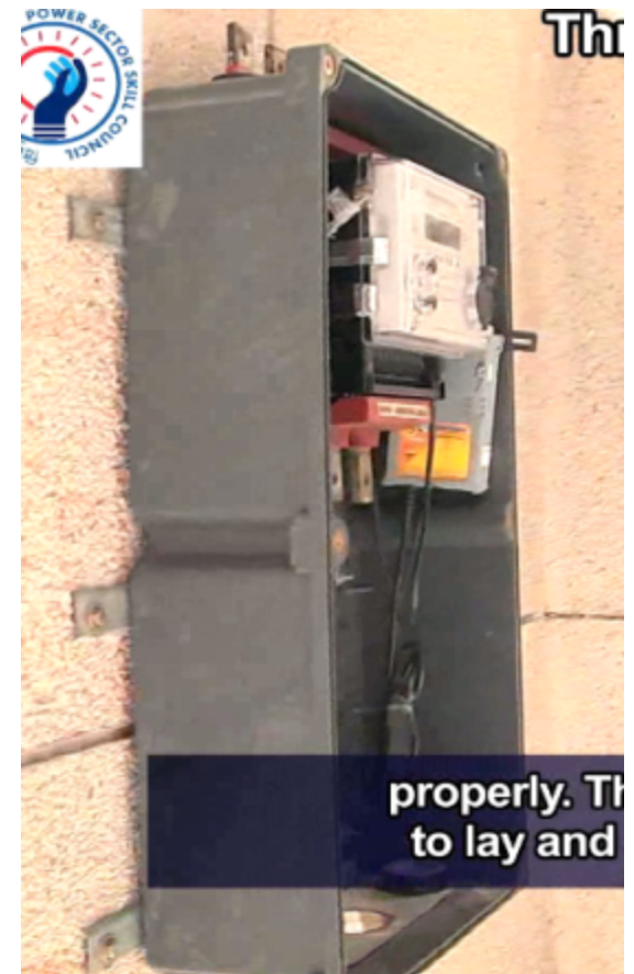
Meter box is properly positioned
