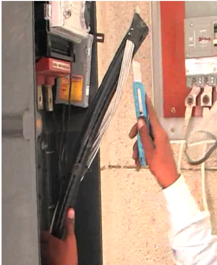
Separation of armoured wires
