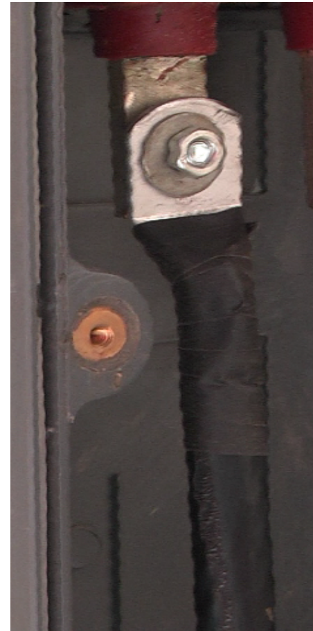
Fixed on the terminal
