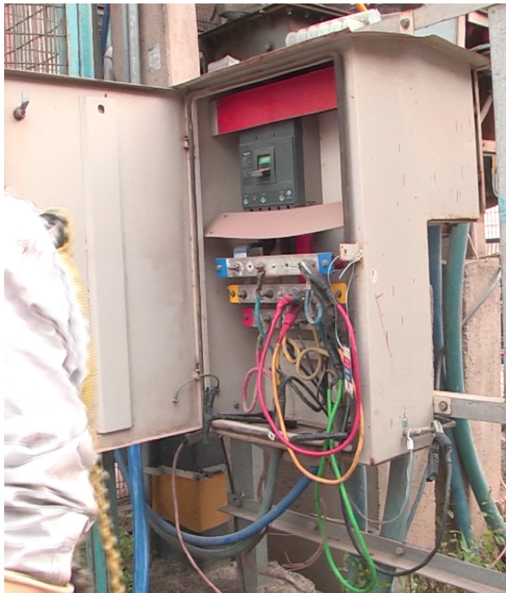
Three-phase MCCB of transformer
