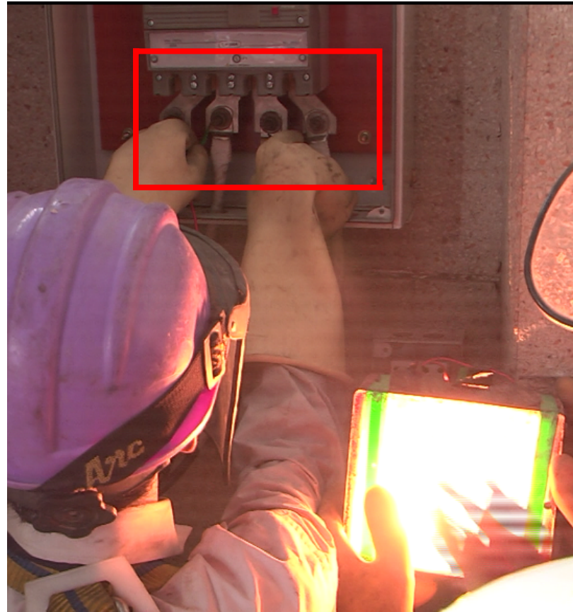
Phase-to-phase checking of sequence 3
