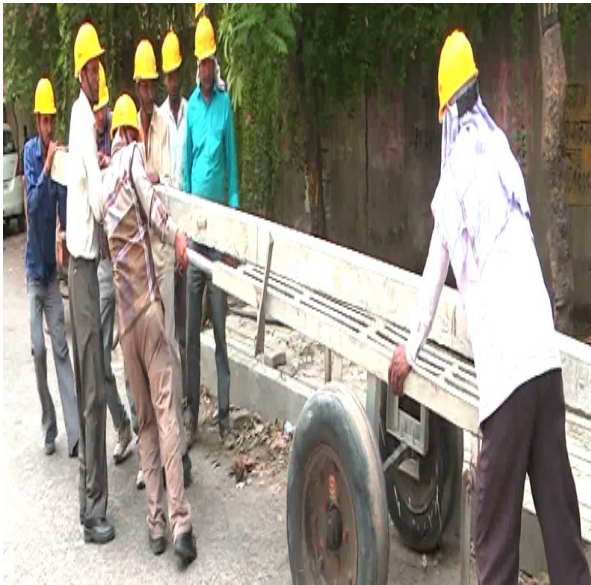
Pole is being pulled by the major axis without tying it
