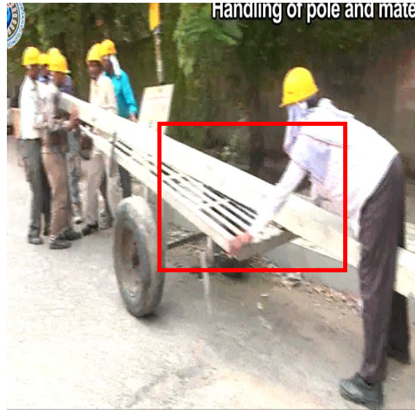
Pole has been wrongly loaded
