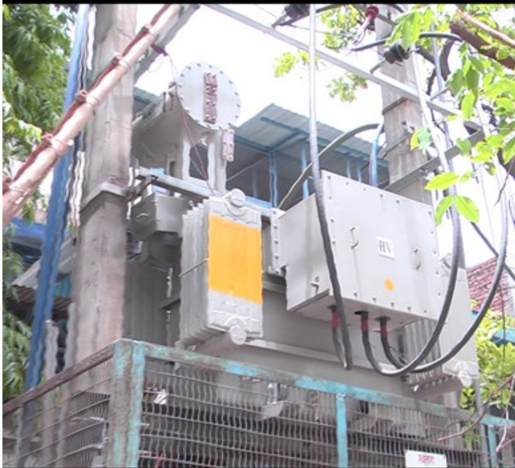
Single core 95 sq mm cable leads are connected on HT side
