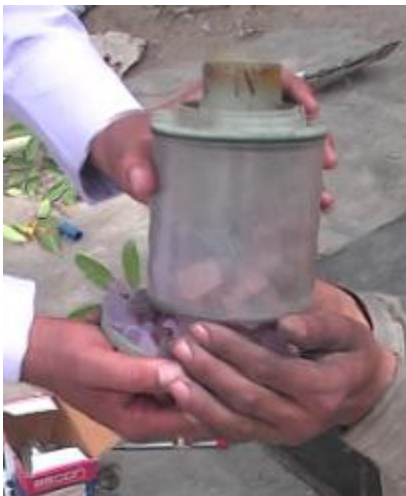
Breather unit of transformer
