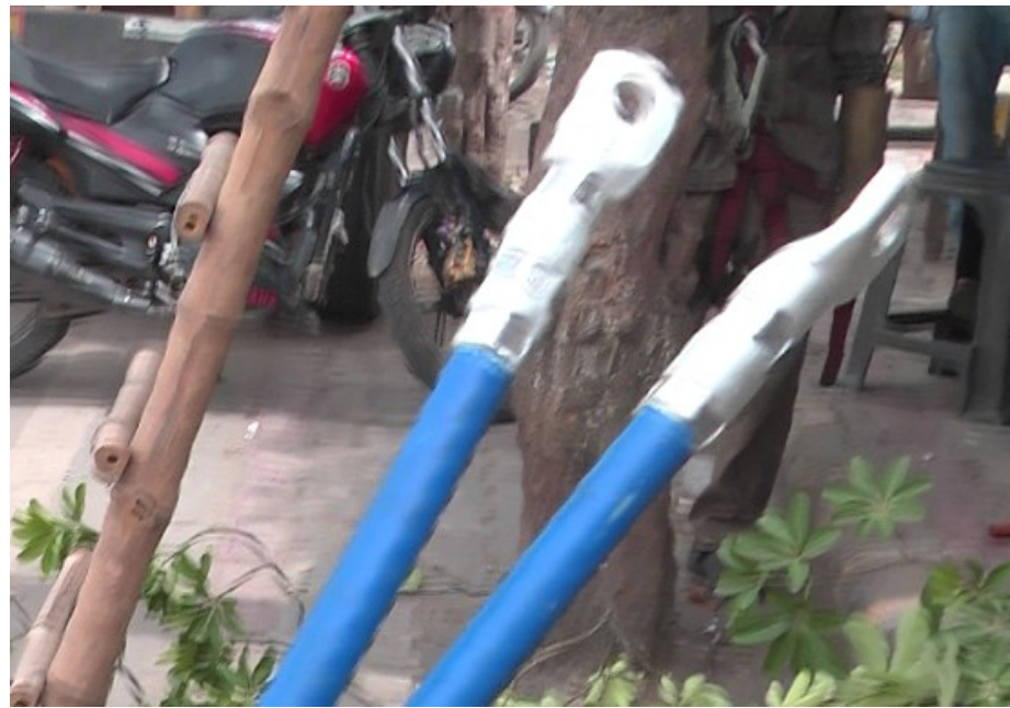
New jumpers to be used for replacement
