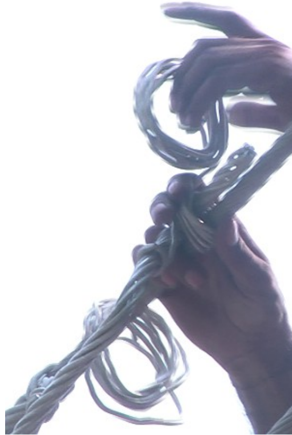
D-Clamp is fixed to avoid loose connections
