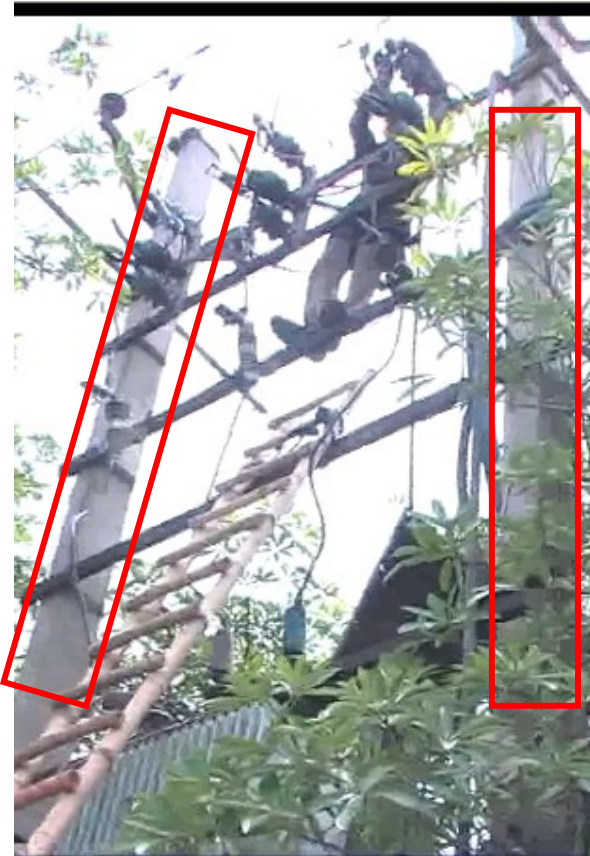
Double Pole (DP) Structure
