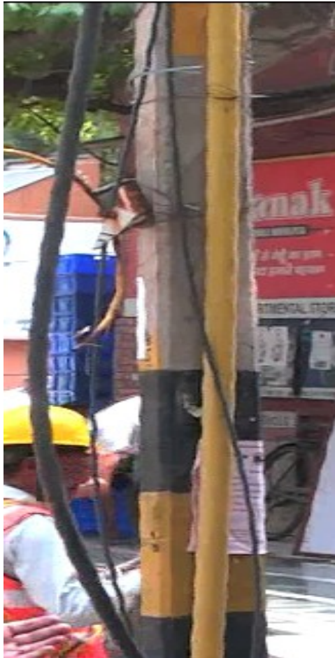
LT Line Maintenance Pole
