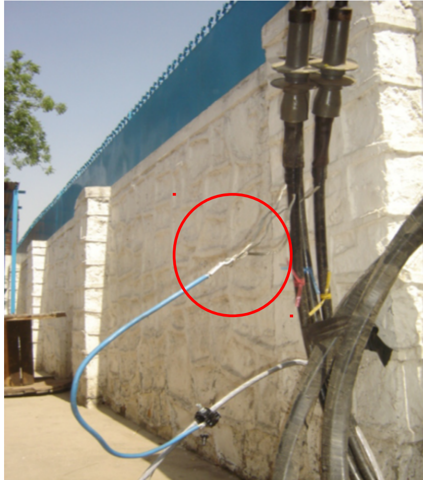
Earthing in HVDS
