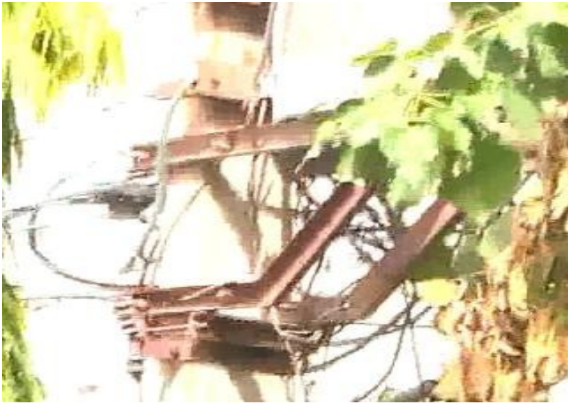
High Voltage Distribution System
