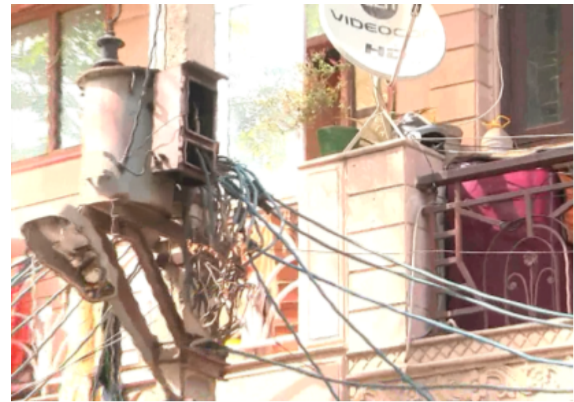
HVDS in Front of Houses
