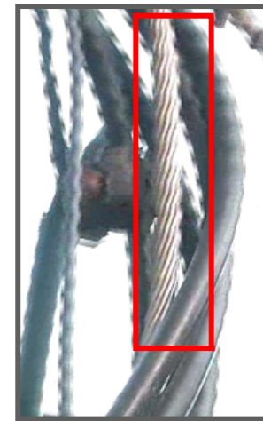
● Messenger cable, the bare one
