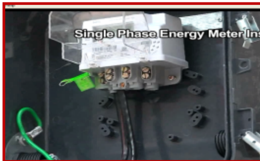
Service line connections
