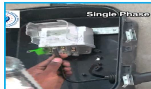
Out going line from the meter terminal
