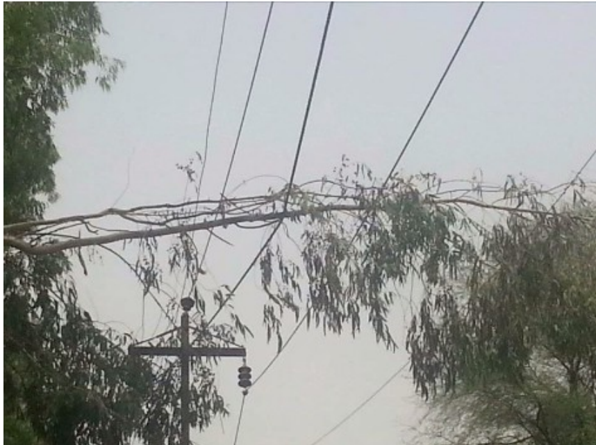
Tree fallen on the HT lines
