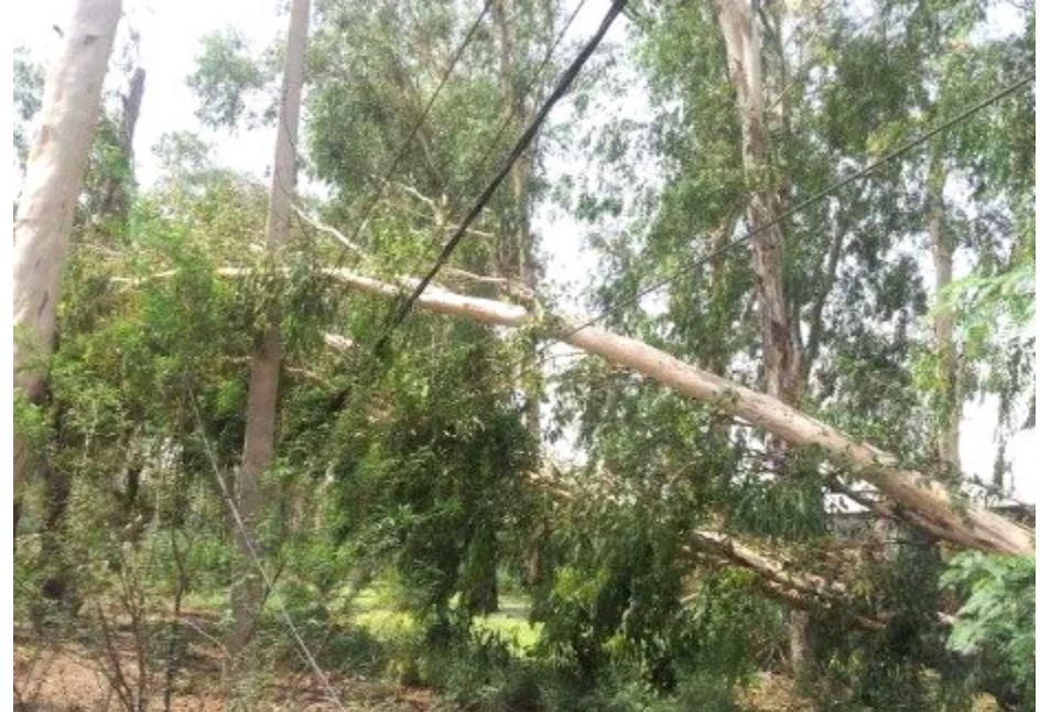
Damaged HT lines due to tree fall
