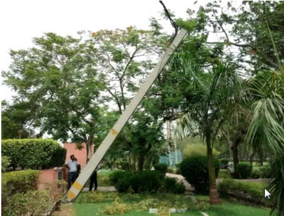
Uprooted PCC pole carrying HT ABC line
