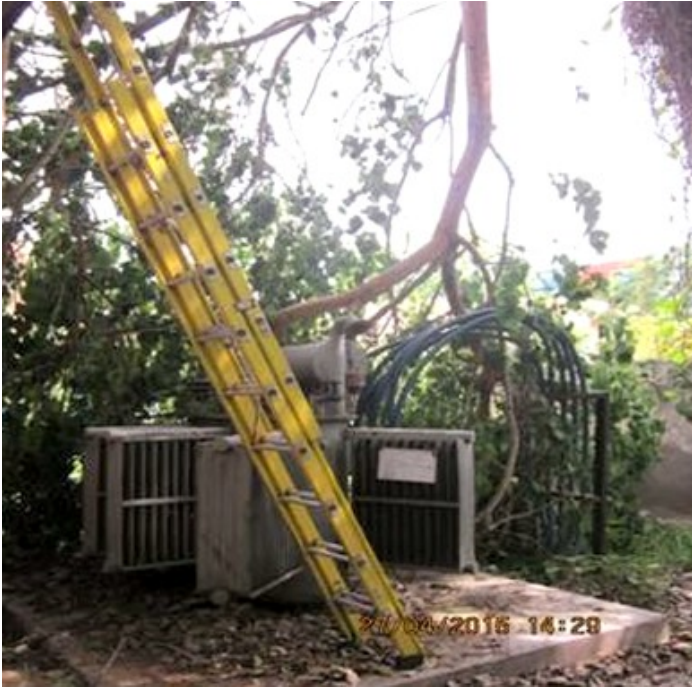
Tree has fallen on plinth mount transformer
