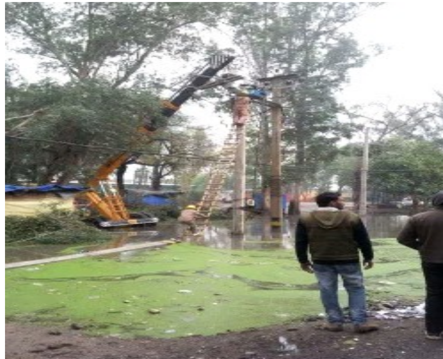
Damaged HT lines in a flood- affected area
