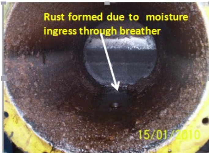
Inside view of conservator tank
