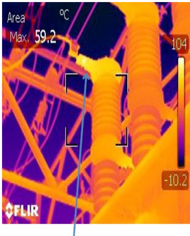
Thermal Imaging Showing Hot Spot
