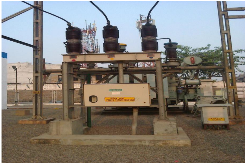
33 kV Circuit Breaker
