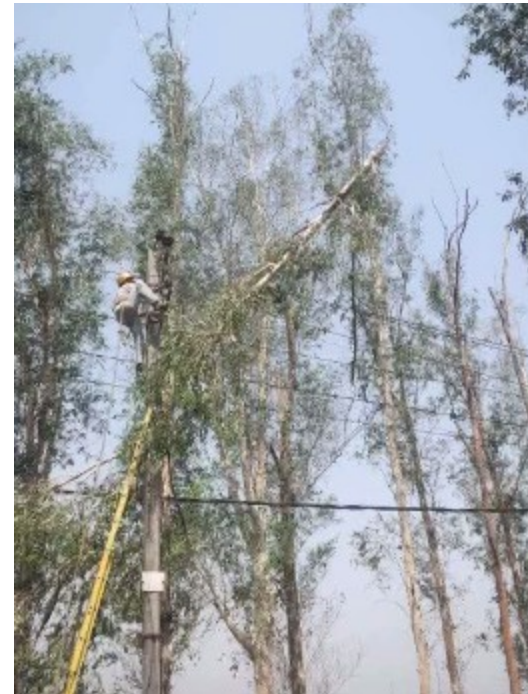
Branch of tree damaged the HT line
