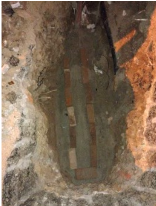
New HT cable joint
