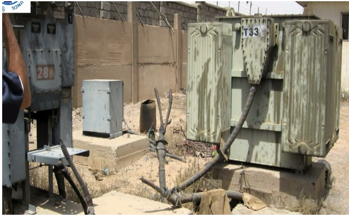
OCP tripping and flash at cable termination
