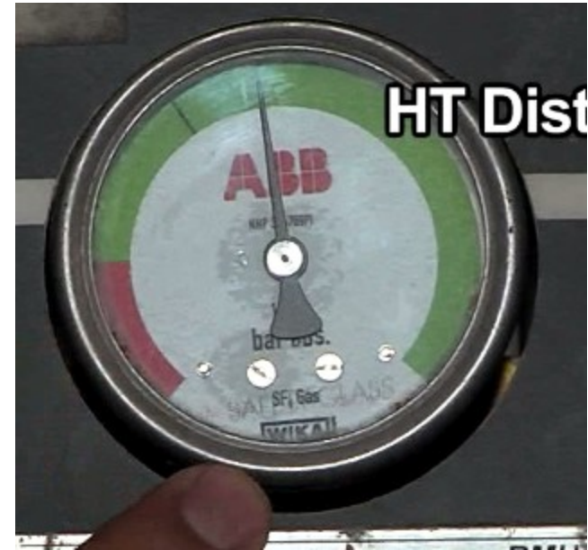
Voltage Presence Indicator System (VPIS)
