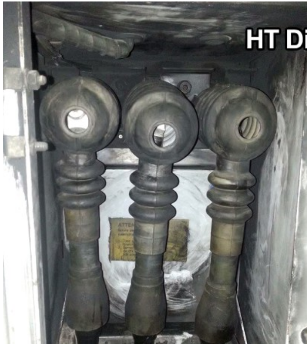
Flash in RMU cable chamber
