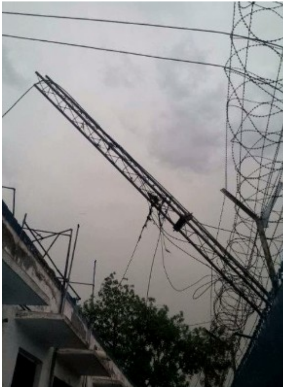
Communication tower uprooted due to a storm
