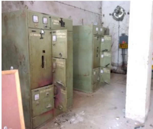
LT switch-board panel
