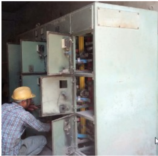
Components of panel about to collapse
