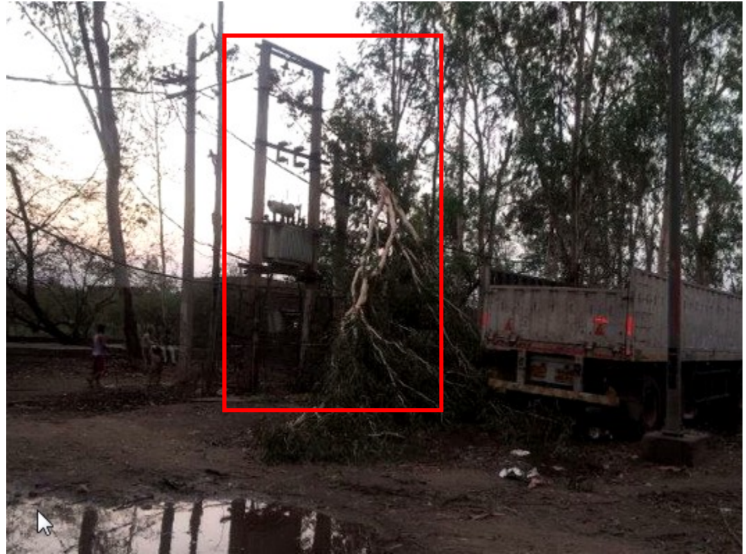
Tree has fallen on the LT lines
