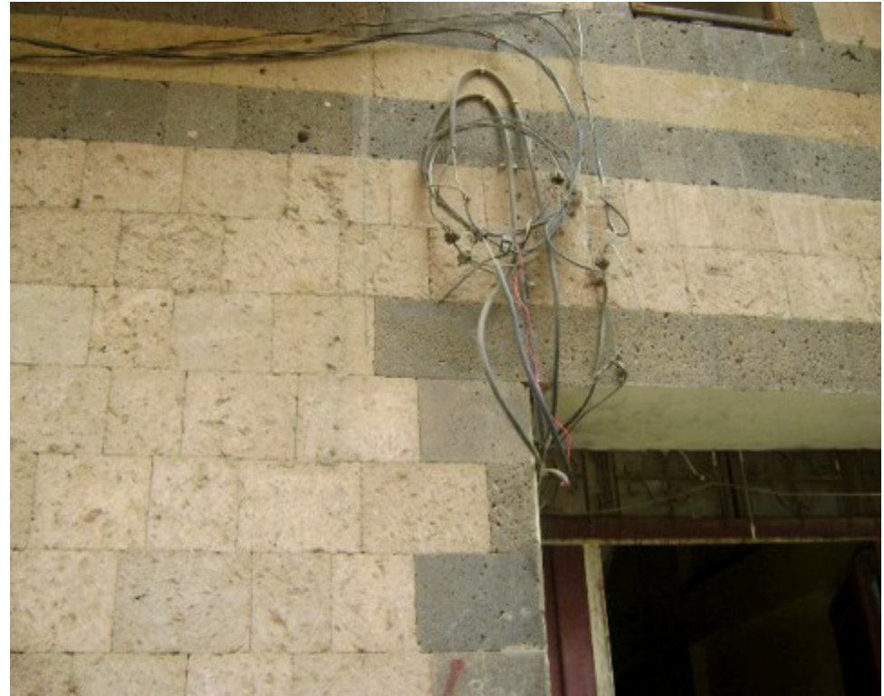
Loose joints in incoming service line
