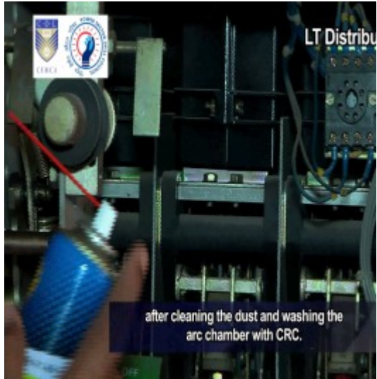
Arc chamber is washed with CRC
