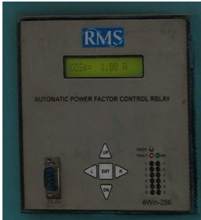
LT control panel in a substation
