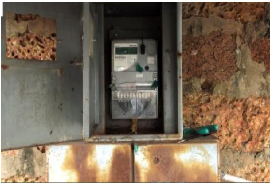
Rat dung on the base plate of meter box
