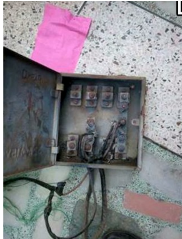
Loose connections and temporary joints in bus bar box
