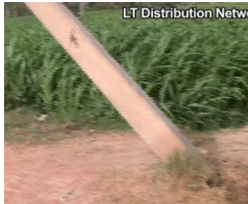
Broken and uprooted LT PCC pole
