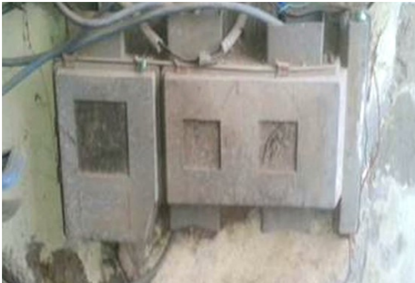
Bus bar box, where service line is connected from the meter
