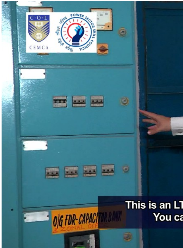
LT control panel in a substation
