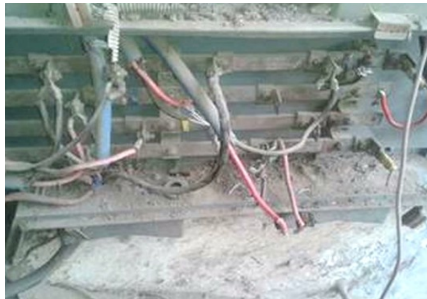
Overheated and damaged outgoing leads
