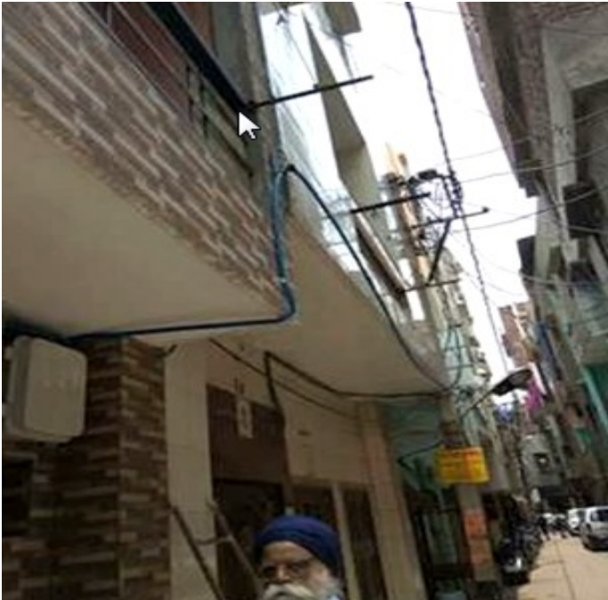
Clamped service cable up to the meter box
