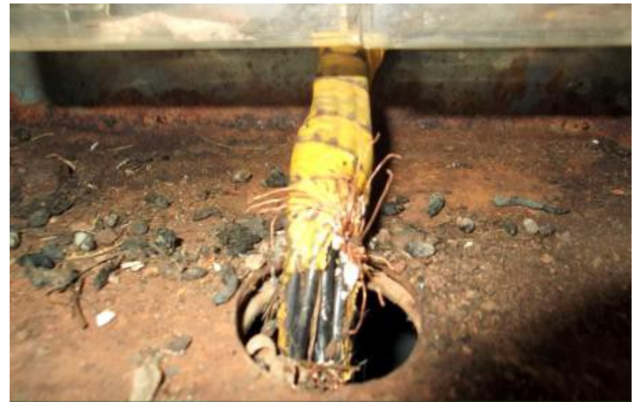
Neutral is missing as rats have cut the neutral wires
