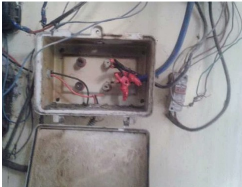
Bus bar strips are missing
