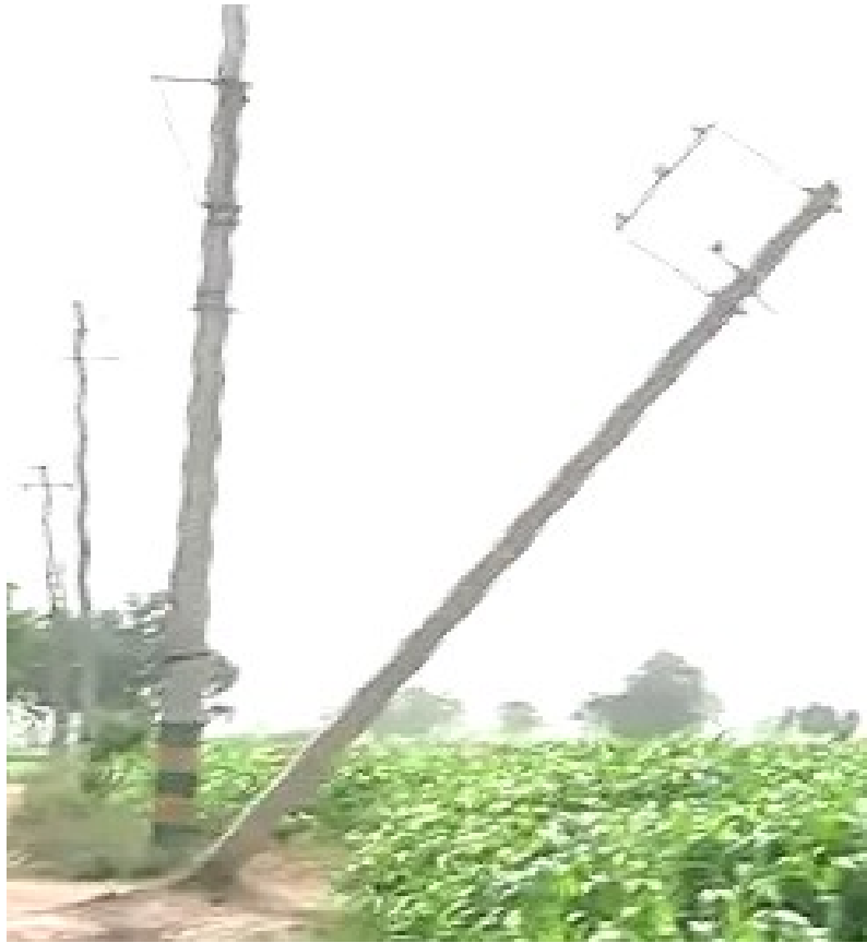
Pole is tilted from its base
