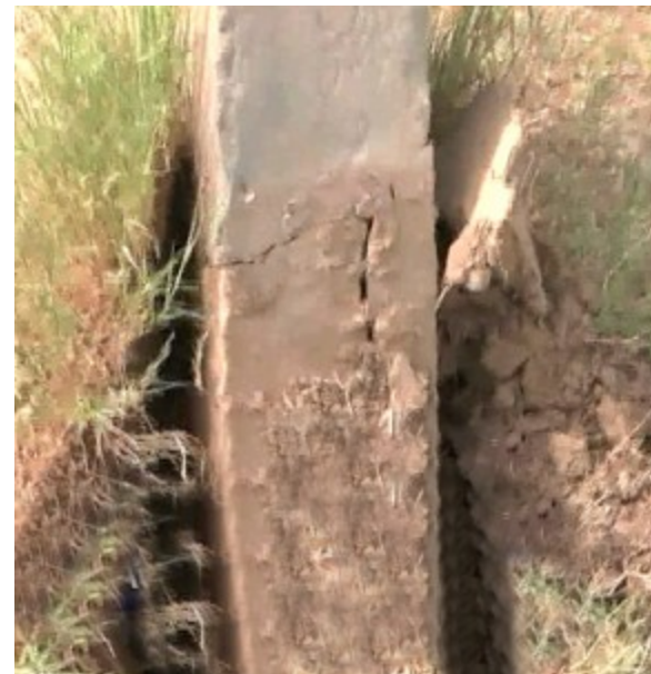
Uprooted LT PCC pole
