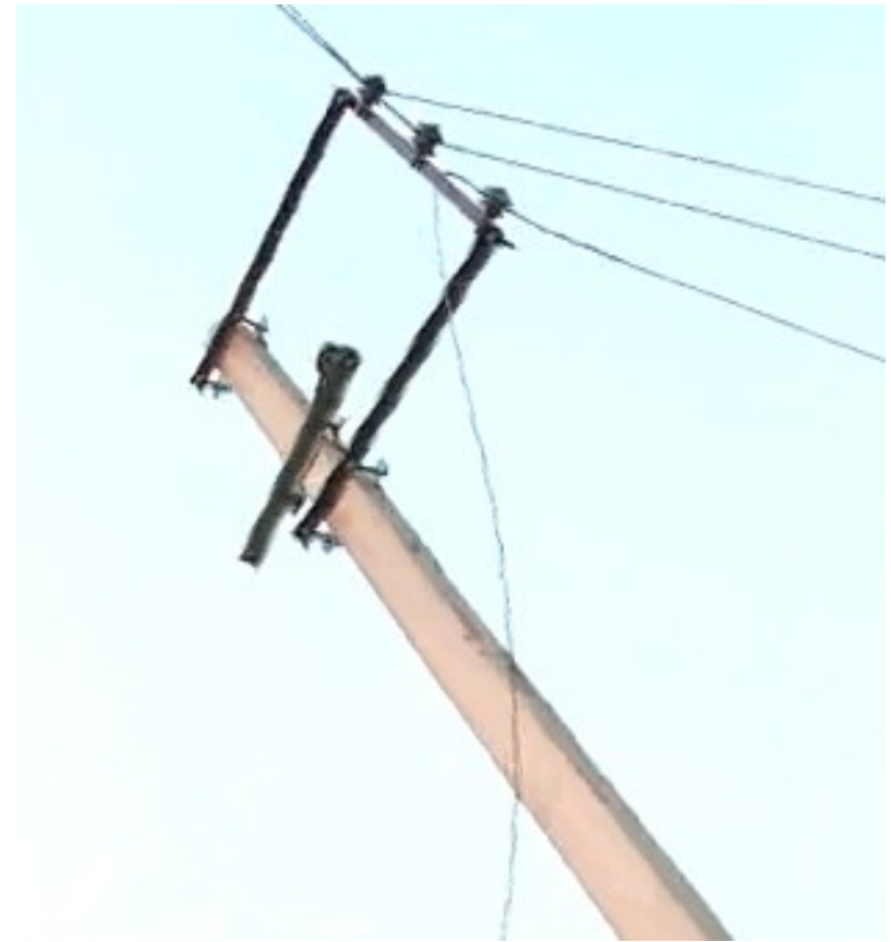
Lower conductor of third phase is snapped
