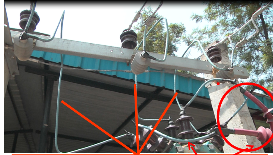
These are connected to the main line and the earthing terminal
