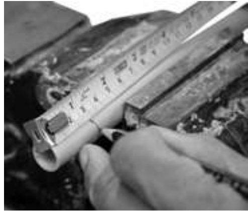
Step 11: Mark 25 mm. on 12 mm aluminum pipe. It is used as a spacer between the members ofscreen
