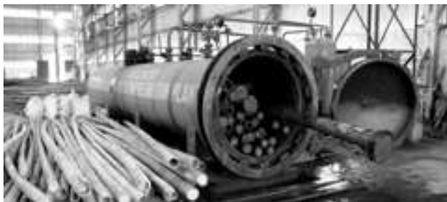
Pressure treatment tank
