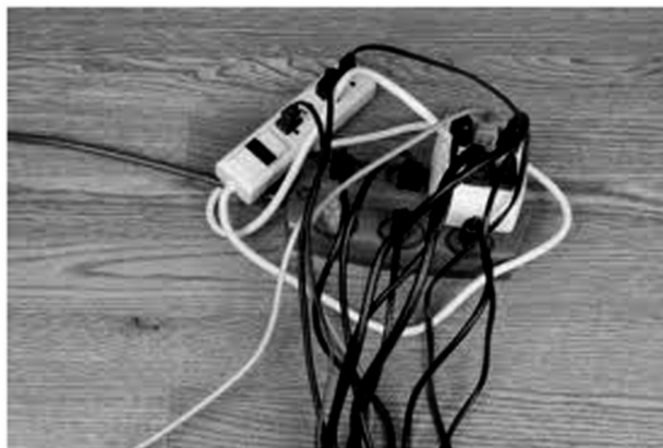
Fig. 11.2: Overloaded power strip.
